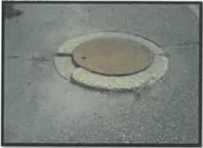
Traffic Signal Handhole
