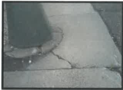
Traffic Signal Pole
